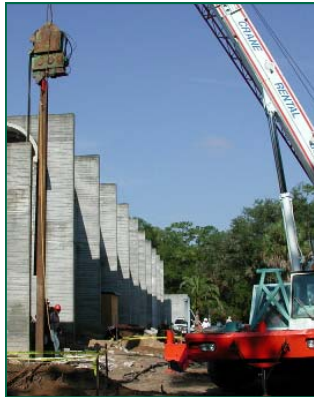
The first beam for the new education towers was lifted into place last Wednesday.
