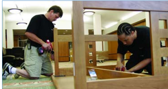
Workers assemble tables for the Stephen C. O'Connell Reading Room in the Lawton Chiles Legal Information Center. The library completed the move to its new facilities in Holland Hall in early August.
